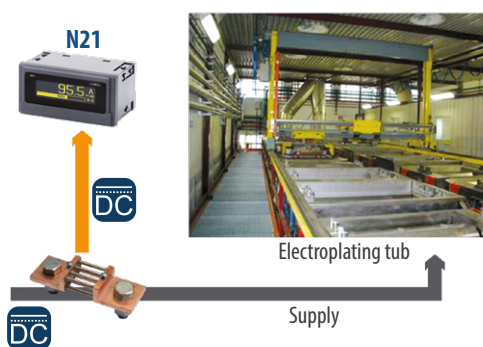
Current measurement in an electroplating plant
